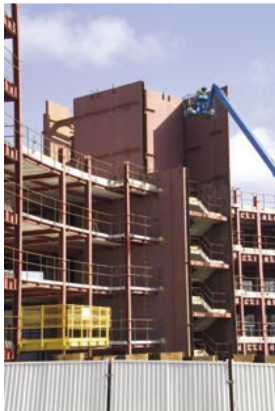
Core panels for the Birmingham 1 project were fabricated to precisely accommodate the building's horizontal curve.
