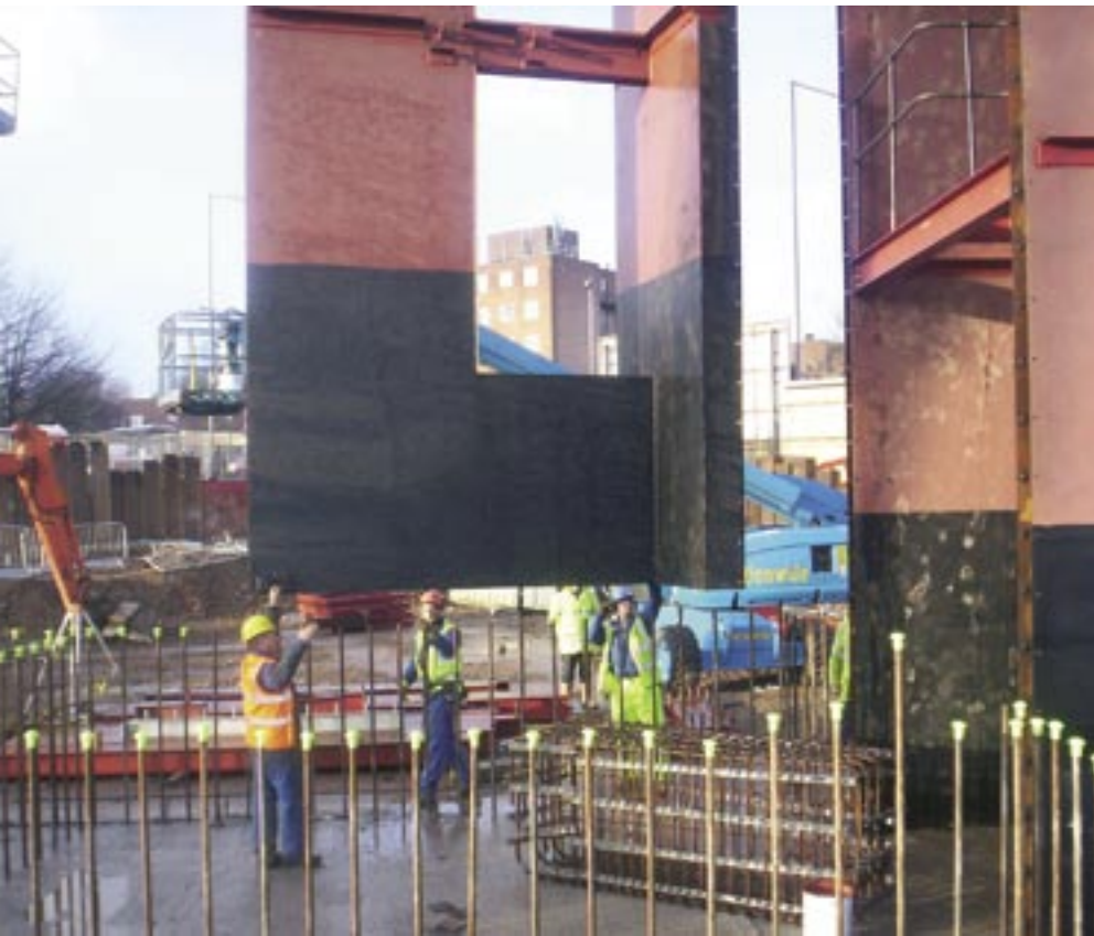
Bi-Steel panels are fabricated off-site and assembled section-by-section to form a steel core. When all segments are erected, concrete is placed between the inner and outer steel plates.
