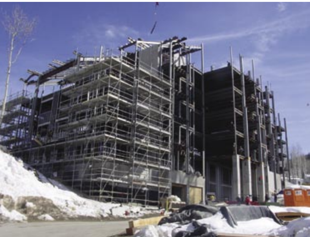
Larger than Grand Lodge, Silver Strike Lodge has two floors of parking topped with six floors of condominiums.
