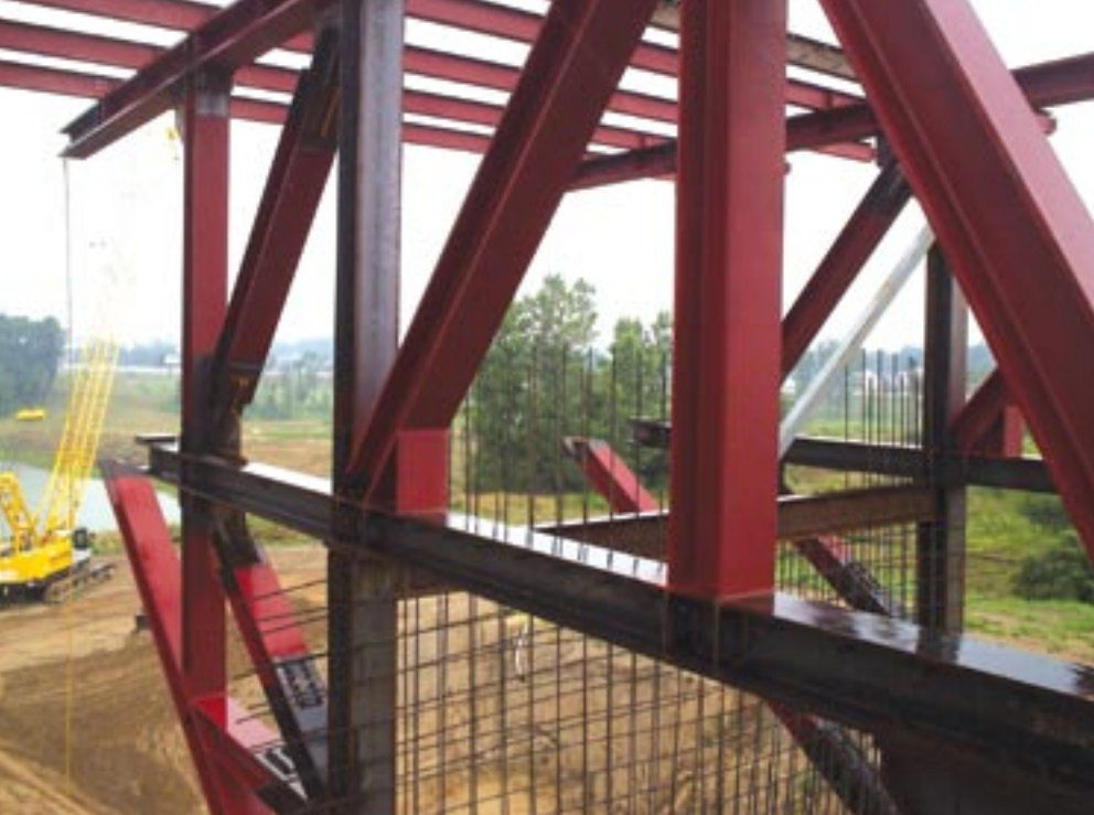
A steel frame sheathed in concrete provides the structural support for the massive cantilevers.
