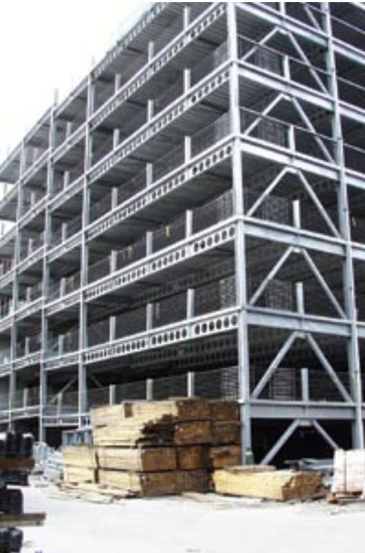
The Delaney Square parking structure in Orlando, Fla. features a galvanized steel frame.
