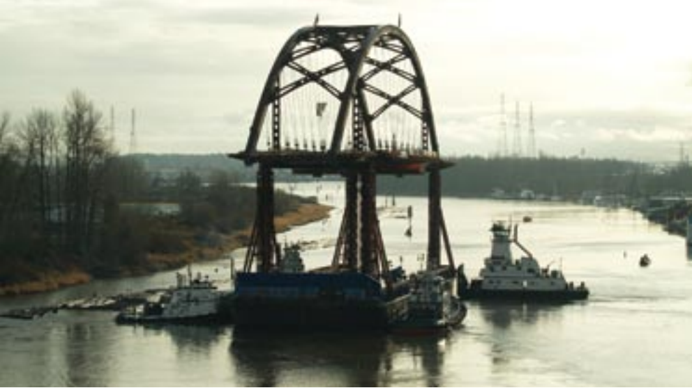
The tied arches and floor system were assembled eight miles from the bridge site and delivered to the site on barges.
