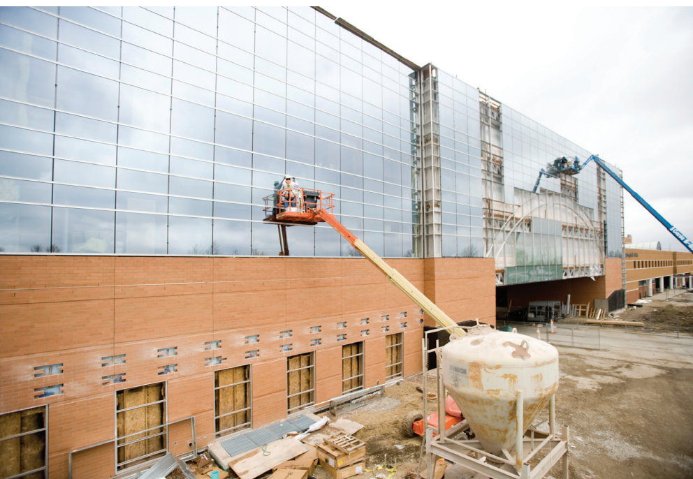
The structural design for this expansion project was driven by an aggressive 21-month design and construction schedule.
