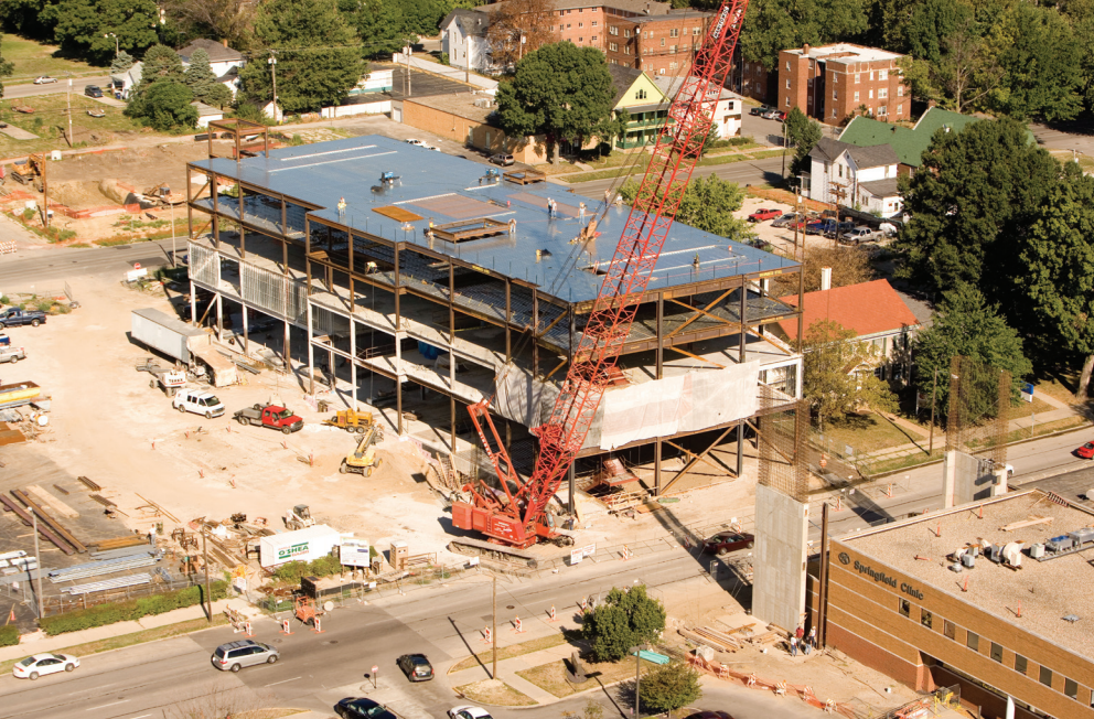
Hanging the curtain wall from the roof structure minimized the vertical movement under applied live loading and eliminated the need for expansion joints between levels.
