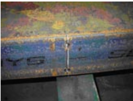
A full-flange transverse crack of a W21x93 taking place during cambering.
