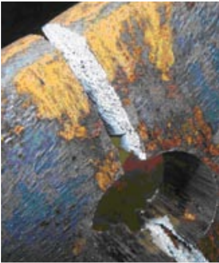
A close-up of a camber crack through a W-shape flange with a punched bolt hole.
