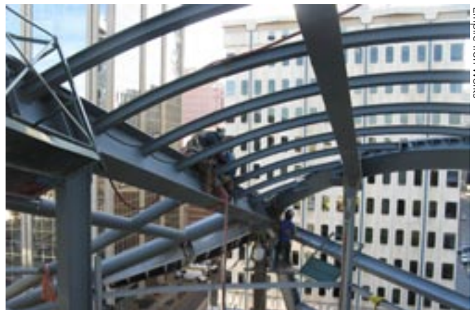
Steel members of all types and sizes bring the unique structure together.
