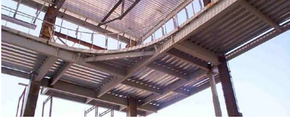
Above: Composite steel cantilevered running track in the Jerry D. Morris Recreation Center gymnasium is supported by composite steel columns.
