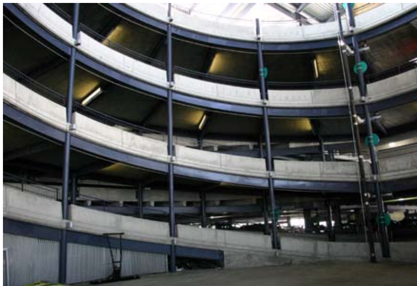
This page: The JetBlue garage at the Portland (Maine) International Jetport uses a steel framework on the spiral ramp to support the floor slabs.
