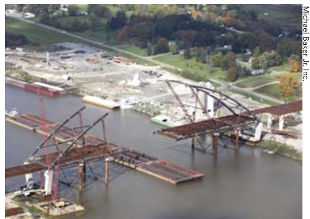
Constructing the networked, tied-arch span of the Blennerhassett Island Bridge over the Ohio River in 2007.
