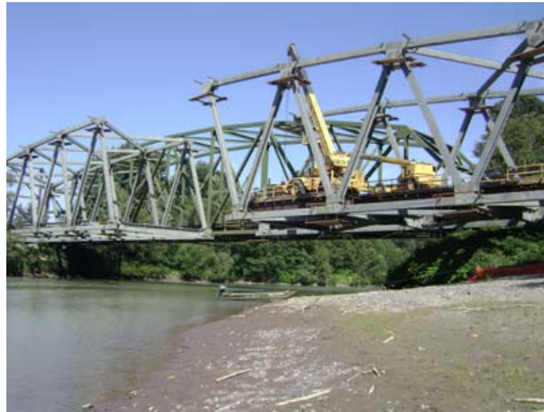
Because access for a large land-based crane was not available on the south shore of the Nooksack River crossing, the anchorage and backstay system had to support the weight of equipment as well as the truss weight.
