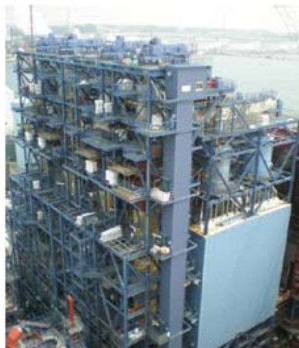
The emissions from the coal-fired Isogo Power station (shown here) are at comparable levels to those from natural gas-fired facilities.
