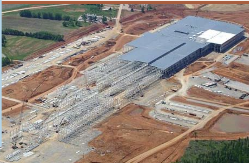
Installation of the initial 19,000 tons of structural steel for this mile-long facility was completed in 17 weeks, a pace that required exceptional planning, coordination and execution. The facility required a total of 21,000 tons of steel, 200,000 bolts, nine miles of crane rail, and three miles of handrail. All photos courtesy of Midwest Steel, Inc.
