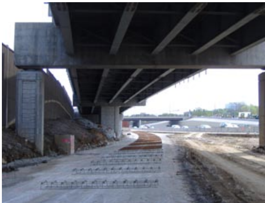
▲ To reduce the height of the bridge by several feet, the steel I-girders were framed in with the concrete cap beams at three of the four interior piers.
