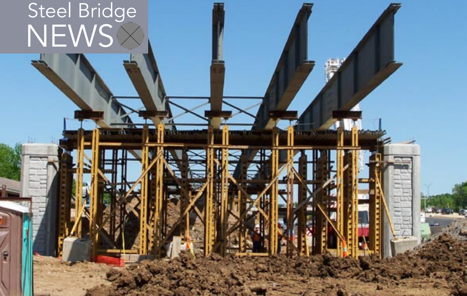
▲ ▼ The steel girders were supported by falsework (above) until the concrete cap beam was cast and cured and post-tensioning was completed.
