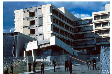
▲ Fig. 1: Olive View Hospital following the 1971 San Fernando earthquake; where a stair tower and the psychiatric wing collapsed.
