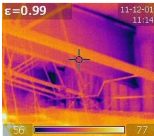
Figure 1: Infrared scan of structural steel balcony beam cantilevering out from a structure.
