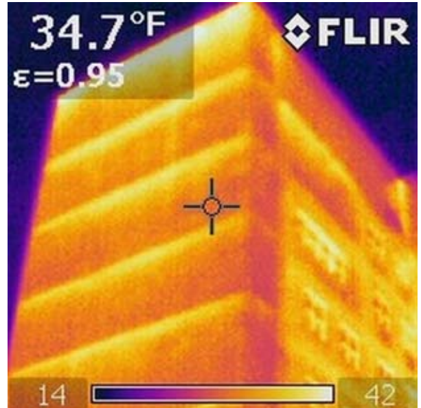
Figure 2: Brick in contact with warm steel shelf angles, which stand out in infrared images.
