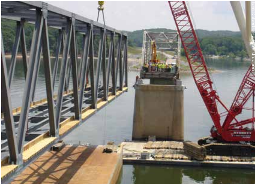
▲ The new section, shown here being lifted into place, weighs approximately 300 tons.
