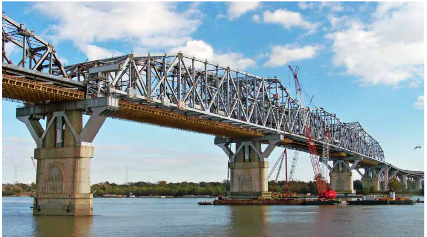
▲ The widening project involves the addition of more than 22,000 tons of new steel.
