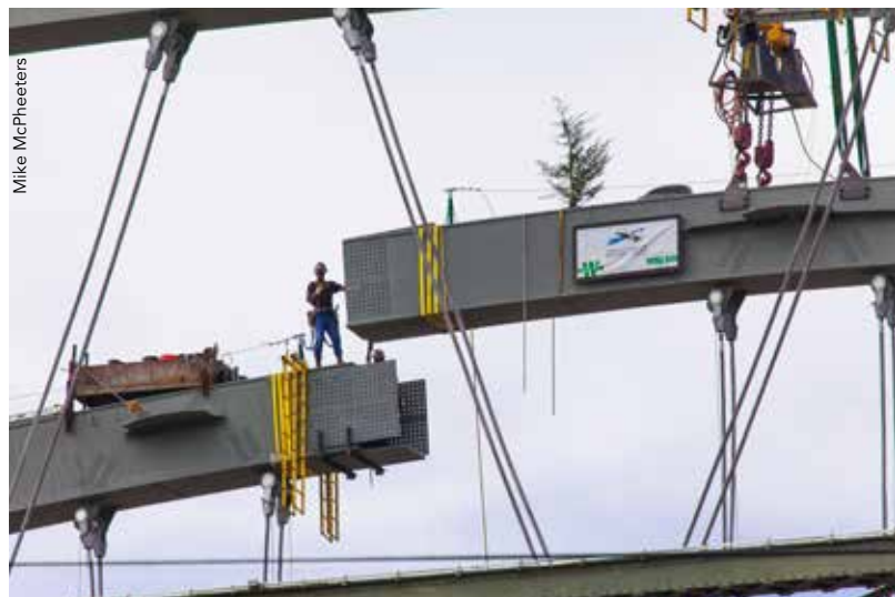
▲ The final arch rib, complete with topping out tree, being lifted into place.
