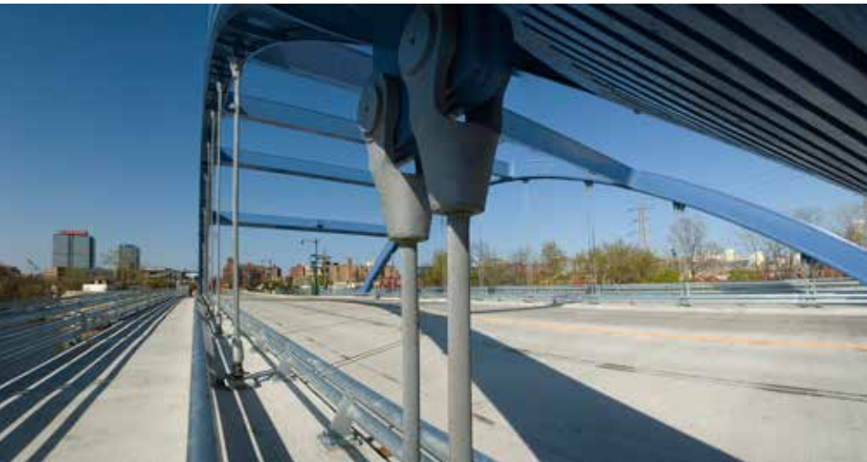
▼ Cable hangers, up close.
