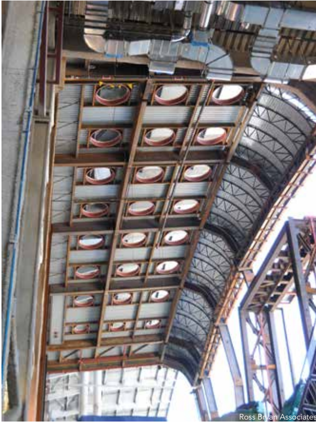
▲ Articulated W30 beams and columns and curved bar joists at the concourse roof.
