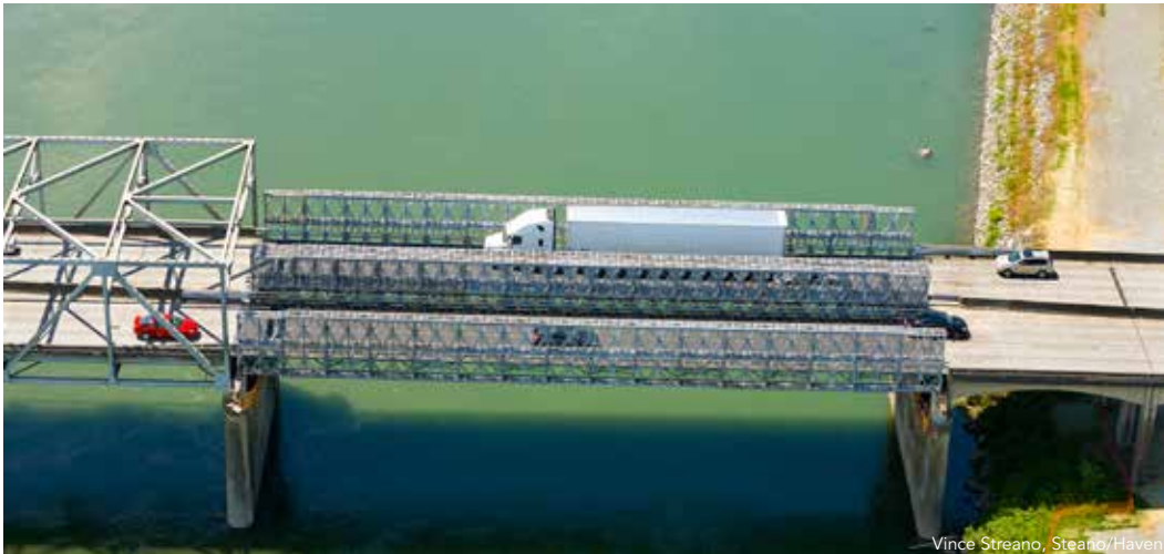
◀ Temporary spans were erected, and the bridge reopened only 23 days after the collapse.
