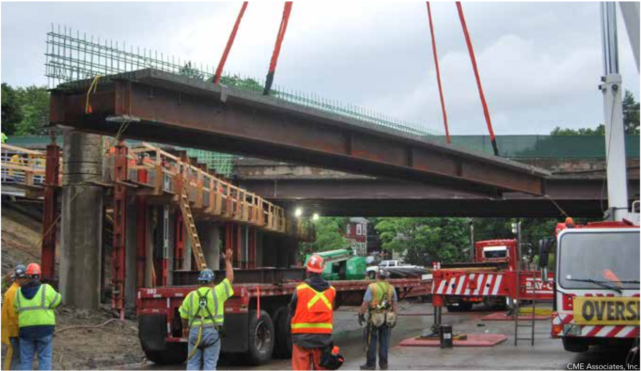
CME Associates, Inc.
