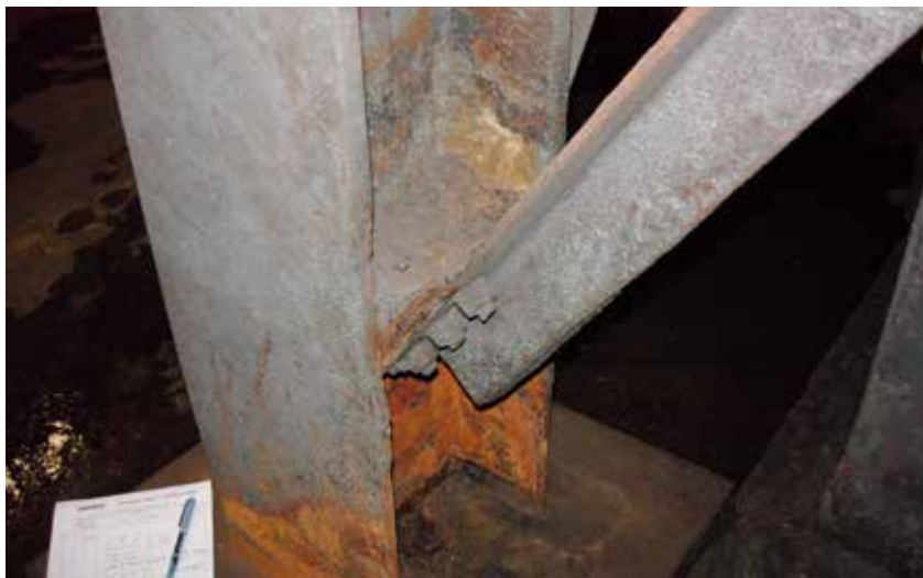
▲ A brace connected with a sloped gusset plate. Note that section loss is apparent while the upper portion of the angle is in good condition.
