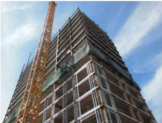
▲ Erection of the 20-story tower, showing the sequence of enclosure on the lower levels during construction of the upper levels.
