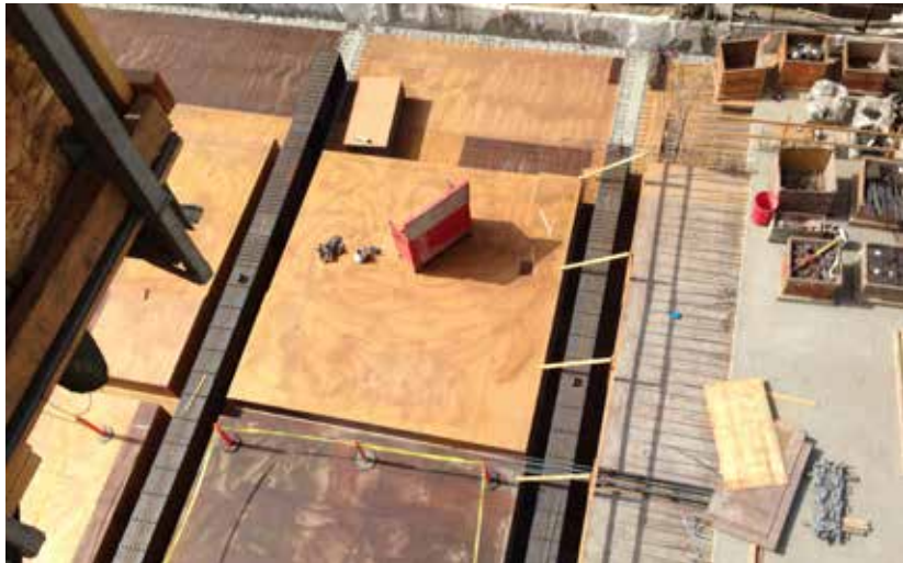
▲ A bird's-eye view of the transfer girders prior to being encased in the podium.
