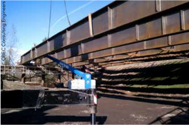
▲ Crews place the girders of the new OR 213 bridge. The girders are fabricated from ASTM A709 Grade 50 weathering steel and are 4 ft, 7 \frac{7}{8} in. deep.
