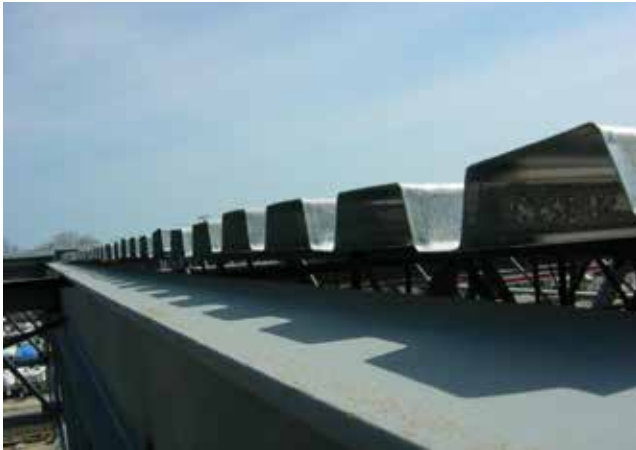
▲ Deck not bearing on un-cambered beam adjacent to cambered beam.
