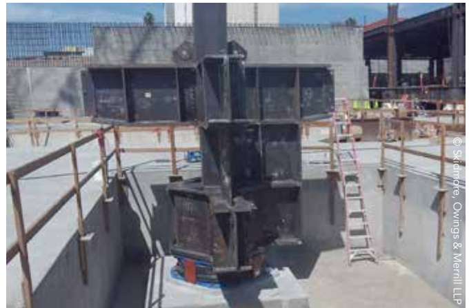
▲ A steel assembly atop one of the seismic isolation devices.
