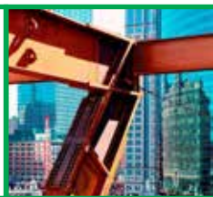
▶ The original truss design involved concrete-filled box columns in order to minimize pick weights, but it was changed to an all-steel option, which proved to be more cost-effective. The W36x925 sloping columns are the largest rolled shapes in the world. All truss connections were bolted.
