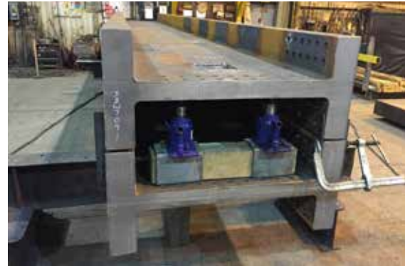
◀ Connecting a type 1 truss diagonal to a node, then a plate girder. All members were test fit on fabricator Zalk Josephs' shop floor.
