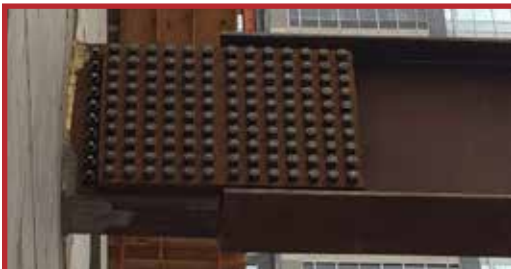
Each connection to the core uses 150 1½-in.-diameter, 15-in.-long A490 SC Class B bolts in double shear. Given the importance of this connection in terms of stability, side plates were added outside of the primary shear planes, effectively creating a quadruple-shear condition and providing a completely secondary load path for the tension forces.
