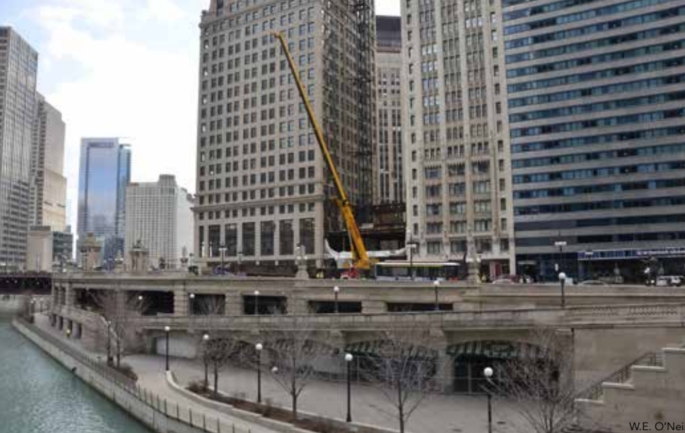
◀ Various views of the double-web plate girder erection. There are four of these girders in all, each framing to a single wide-flange column and transferring the load of the 18 floors above the ballroom level.
