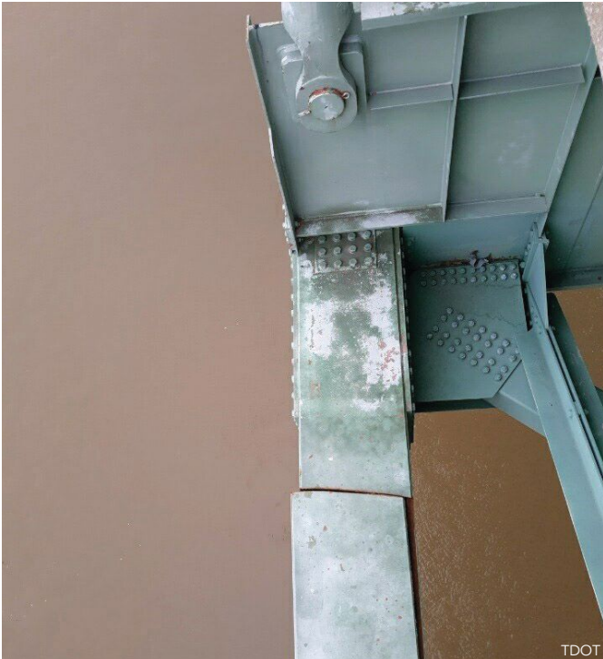
below: The cracked member discovered in the Hernando De Soto bridge in May 2021.
