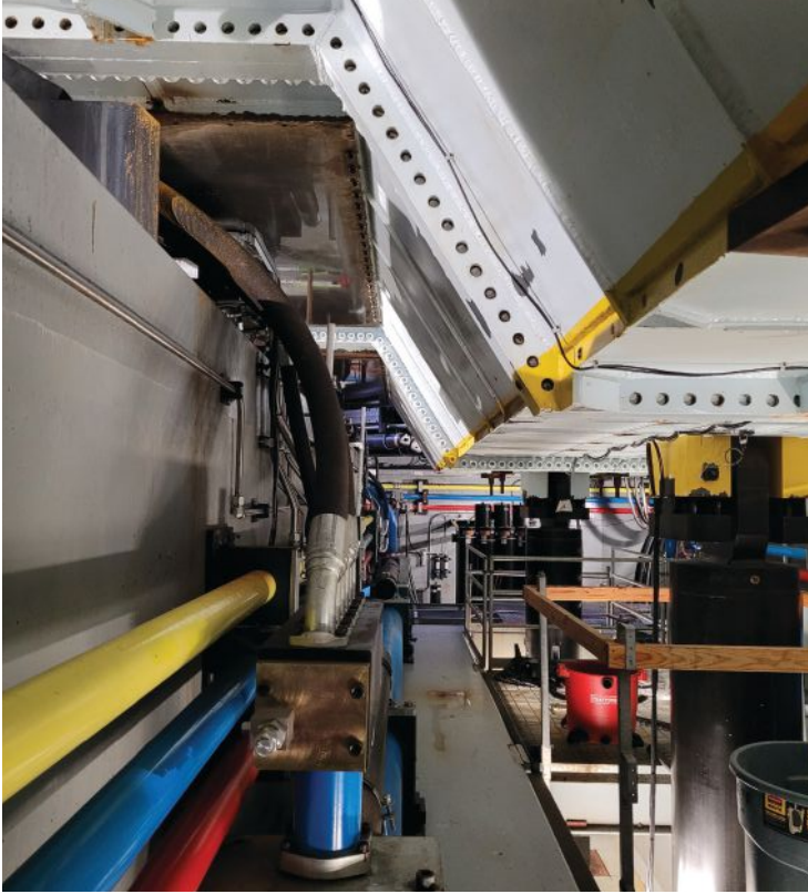
above: Standing in walkway under the shake table. The trapezoidal profile of the platen, the flexible hoses for the low-pressure return of hydraulic fluid from the vertical actuator to the large blue pipe, and two of three hold-down-struts are visible. The hold-down struts provide overturning moment capacity for the shake table.
