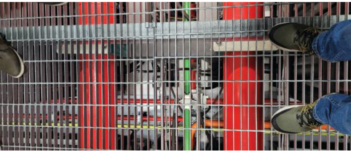
above: The view looking down at the piping beneath from the catwalk in between the accumulation system. The large (12-in. diameter) red pipes carry high pressure hydraulic fluid from the accumulators to the servovalves of all actuators.
