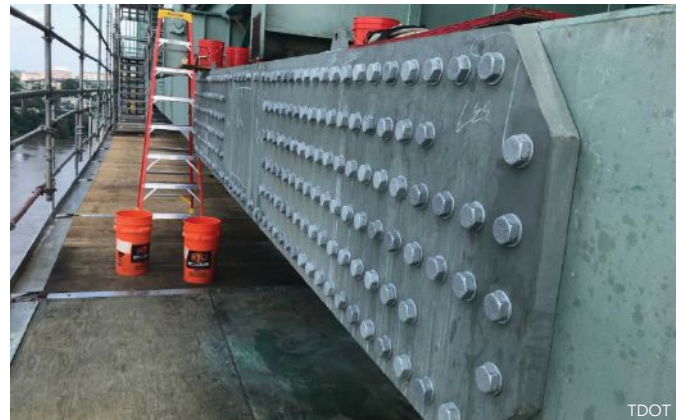
below: A newly installed plate after the last phase of the repair.
