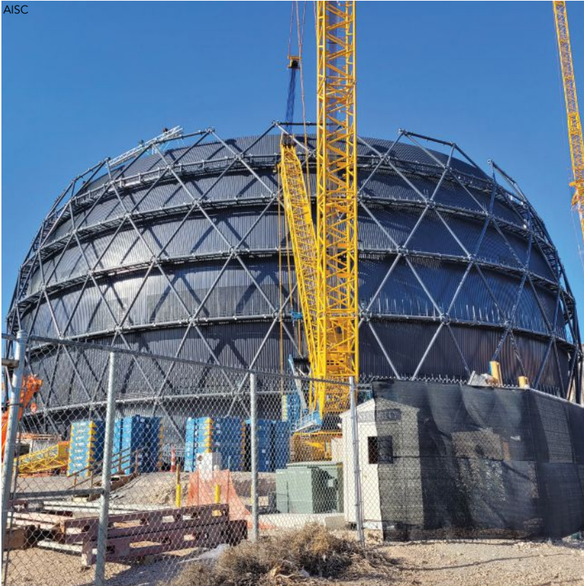
below: The two principal drivers of the Exosphere's design are the angular geometry provided by the nodes and the lengths of the members that frame between the nodes.
