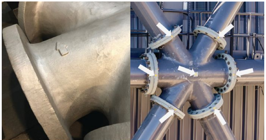
Erector-friendly features incorporated into the cast nodes included "up" arrows for rapid bent assemblies and metrology marks to aid in geometric control and monitoring during construction.
