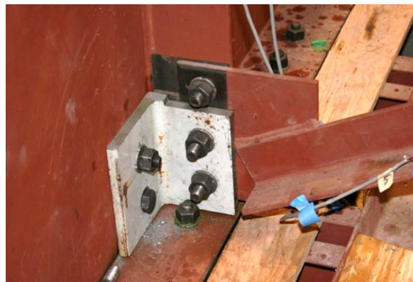
Figure 15. Retrofit measure 6: (a) Schematic of retrofit 6 (interior view); (b) Maximum principal stress contours in the web gap region with the angles removed from view; arrows point to point of highest maximum principal stress along HSS Paths 1 and 2. Cracks were modeled with XFEM and contour integrals. (c) Photograph of interior side of girder with stiffener-to-web angle and backing plate retrofit
