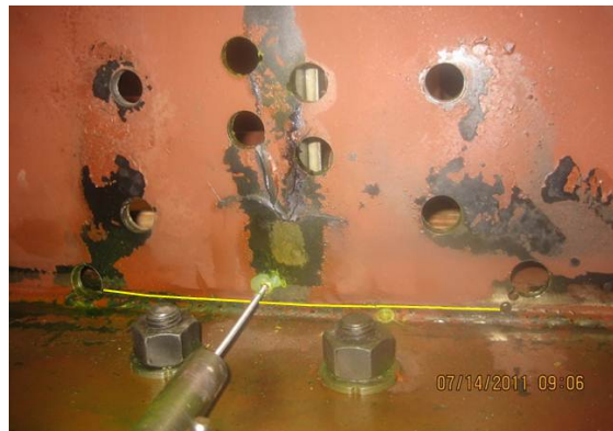
Figure 9: Retrofit measure 1: drilled crack-stop holes (a) Schematic of drilled crack-stop holes, where redlines represent hot spot paths; (b) Maximum principal stress contour plot (cracks modeled explicitly); arrows point to point of highest maximum principal stress along HSS Paths 1 and 2; (c) Photograph of cracking pattern on fascia side of girder. Horseshoe-shaped cracking is visible, horizontal crack has been
