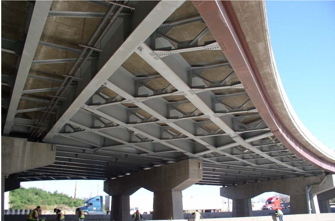
Figure 10: View of curved infill framing area between two orthogonal regions of conventional parallel stringer framing in one of the ramp flare areas of a SPUI bridge structure.
