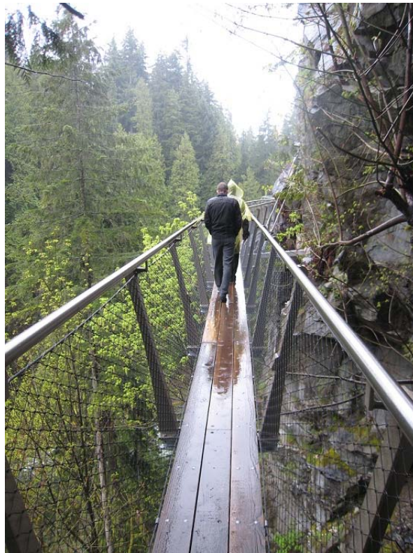
Figure 7. Typical walkway and handrail system.
