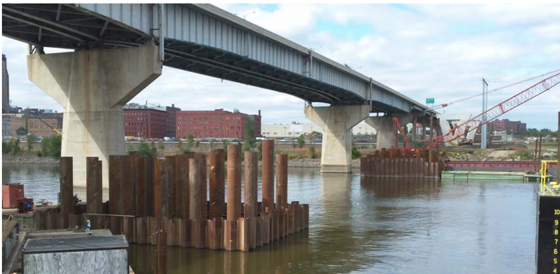
Figure 15 - River pier construction is well underway and scheduled for completion in Spring of 2012.
