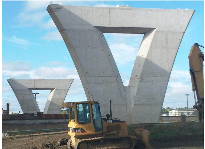
Figure 13 - Strength and shape of approach form compliments trapezoidal tub style and site context.
