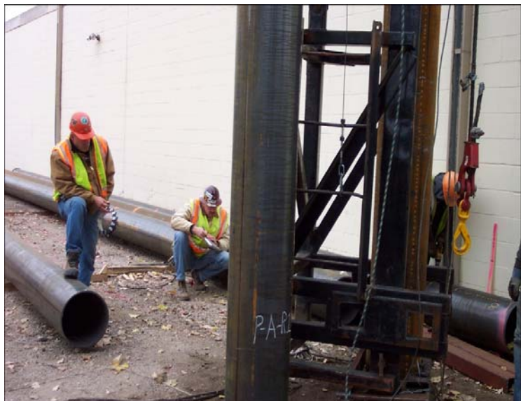
Figure 3 - MnDOT conducted a pile test program in preliminary design to capture significant cost savings in the final design.
