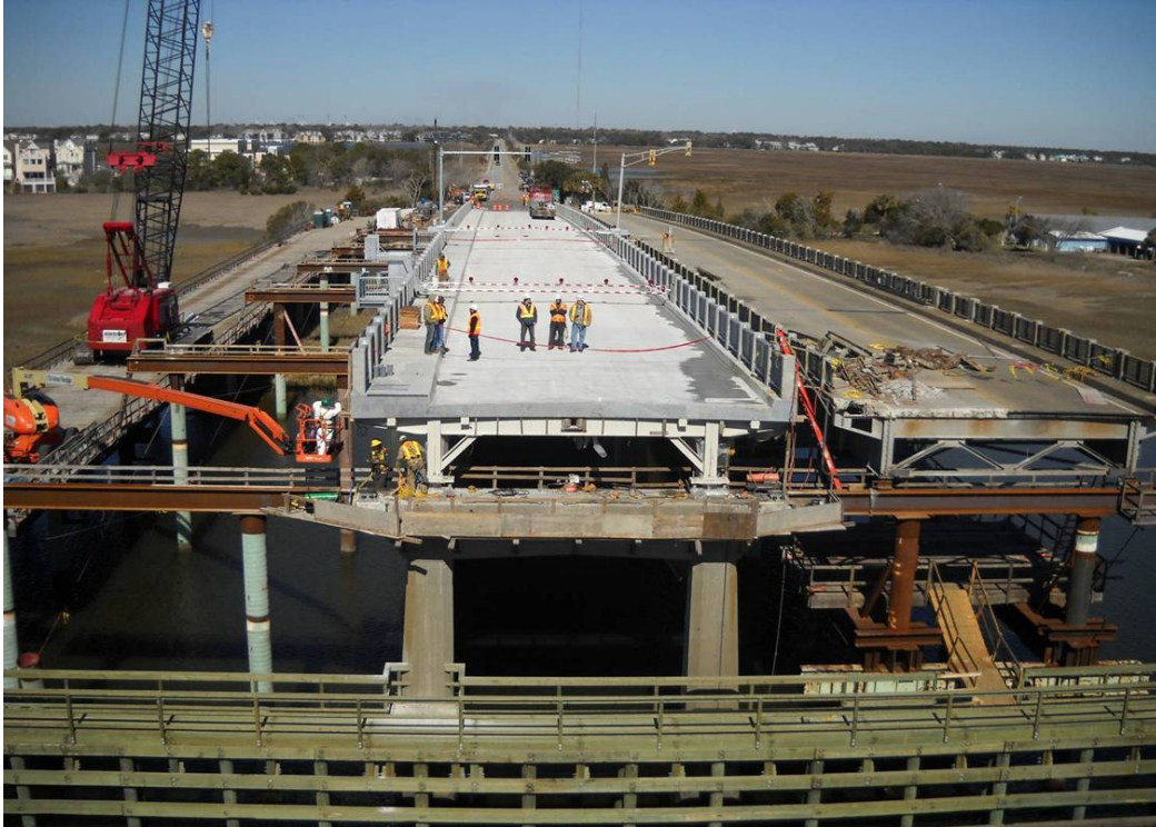
Figure 16: North Rest Pier looking North showing temporary bents and crane trestle. New Approach spans are on the existing substructure and the old approach spans have been moved to a temporary bent ready for demolition.
