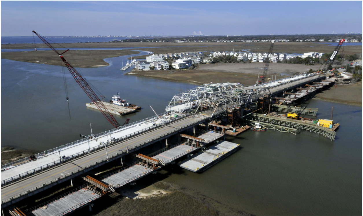
Figure 20: Project site showing old bridge in service and new bridge ready for the move onto the existing substructure.
