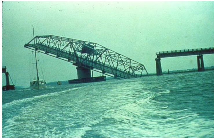
Figure 2: Ben Sawyer Bridge after Hurricane Hugo.
