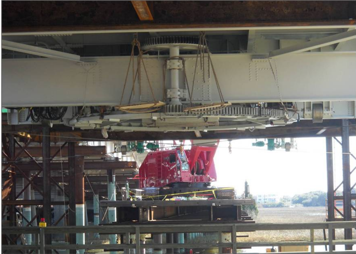
Figure 19: Swing span floating into position over pivot pier. Note all machinery including the rack and pivot bearing is assembled to the swing span.
