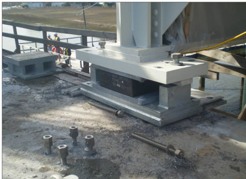
Figure 6: Typical Approach Span Isolation Bearing.
