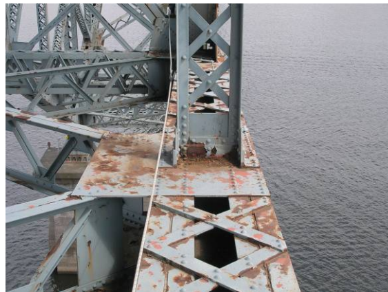
Figure 2. Section losses of Ross Island Bridge in Portland, Oregon
