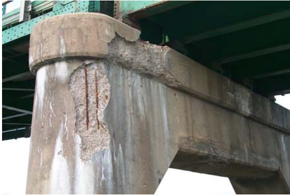
Figure 2: Existing substructure deterioration
