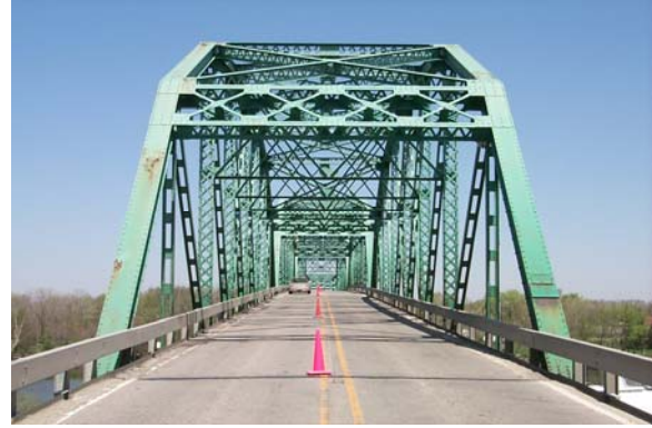
Figure 3: Functionally deficient bridge width
