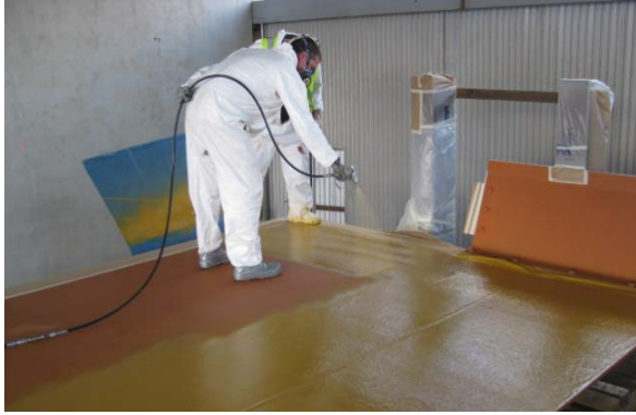
Figure 5: The first layer (1.5mm d.f.t) being sprayed over a primed section of ballast tray. The ballast tray sections were later assembled on site and the site welds were locally abrasive ballasted, primed and protected by 3mm d.f.t elastomeric membrane.
