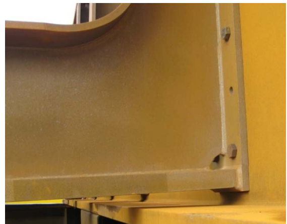
Figure 8: Close up of the cross beam and up stand connection during trial assembly. Note the 50mm clearances between the underside of the cross bottom flange and the top of the main girder bottom flange to prevent debris accumulation and to promote airflow to prevent permanent wetness.
