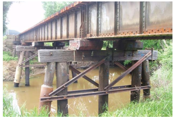
Figure 1: A typical KiwiRail railway bridge subject to high levels of maintenance and inevitable replacement. These bridges feature Steel Plate Girder (SPG) spans and hardwood timber piers often exceeding 80 years of age.
