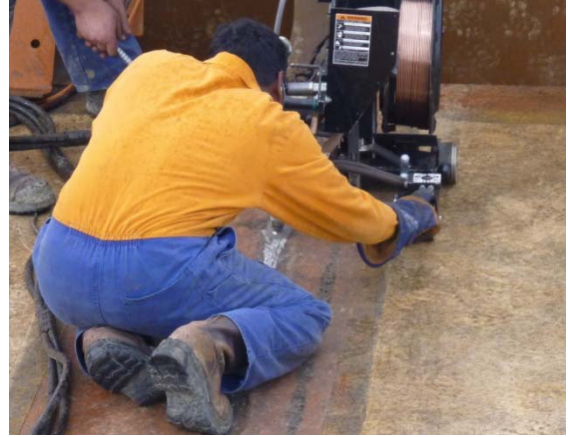
Figure 6: Two adjacent ballast tray sections being site welded. The workshop applied elastomeric membrane coating stops short of the weld. After site welding is complete the weld is abrasive blasted, re primed and coated with a double layer of the elastomer which seamlessly adheres to the shop applied membrane.
