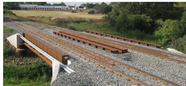
Figure 3: Br 312 NIMT featuring two single track spans each 14m long and weighing 30 tonnes. The track centres are 5m apart.
