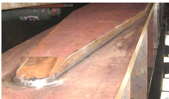
Figure 9: Curtailed top flange doubler plate detail in recognition of reducing moments away from mid span.
