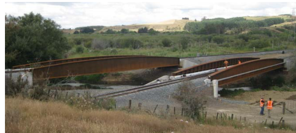
Figure 2: Br 300 (left) and Br 299 (right) NIMT over the Mangatawhiri River near Kellyville, New Zealand. Each BTPG span is 36m long and weighs 150 tonnes.
