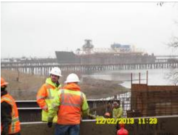
Figure 10 - Mill Creek Bridge construction in a tidal area of the Pacific Ocean.
