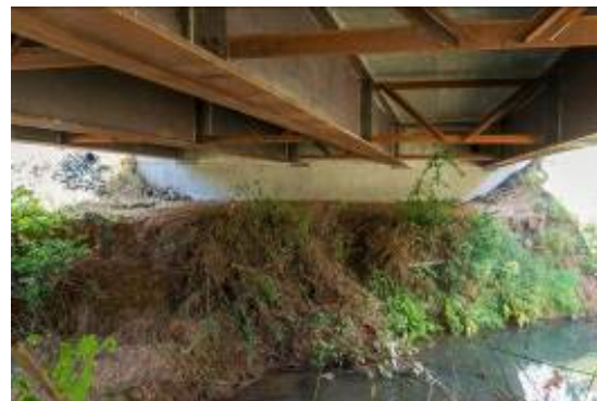
Figure 1 - Grade 50W K-frame connected to ASTM A1010 connection plate with type 3 bolts.
