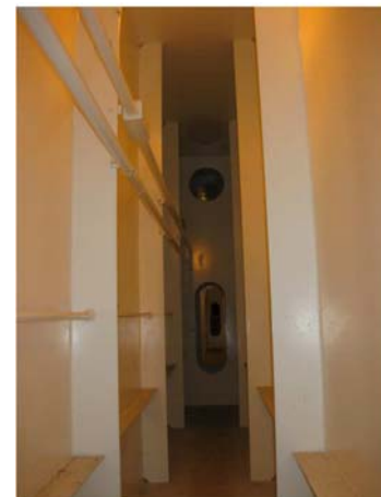
Figure 3: Inside view of the 14' tall x 4' wide - transversely and longitudinally stiffened tie girder of the Hoan Bridge, courtesy of F. Russo (Michael Baker International).
