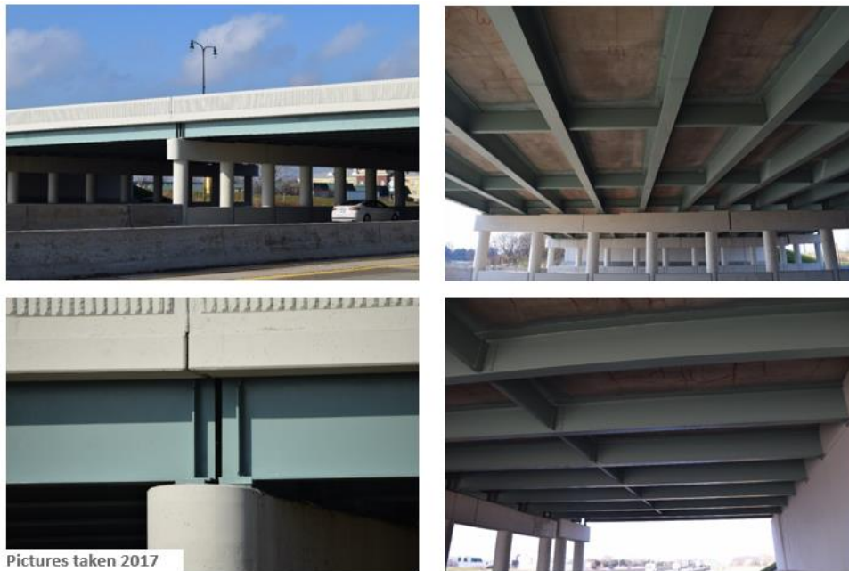
Figure 6. Michigan DOT; West Road over I-75 in Woodhaven, MI. Repainted with PAS system in 2017.
