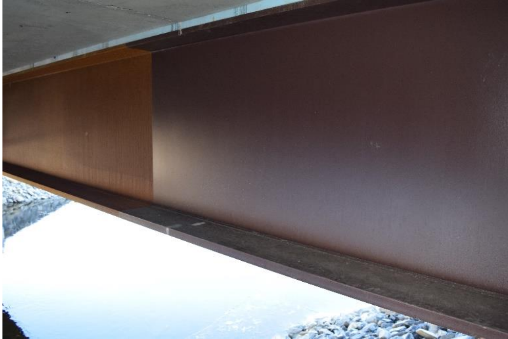
Figure 10. Close up view on one of the painted beam ends.
