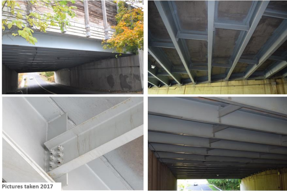
Figure 5. Connecticut DOT; I-75 over Starr Ave in Danbury, CT. Repainted in 2002 with PAS system. After 15 years in service, <0.1% rusting across entire structure.
