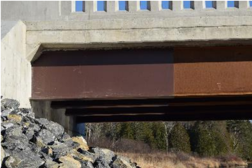
Figure 9. Close up view on one of the painted beam ends.
