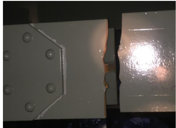
Figure 1: Fractured Truss Chord
