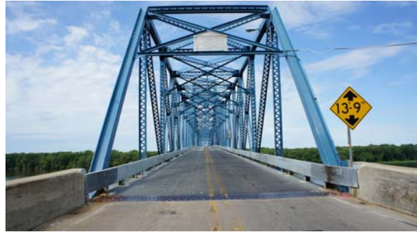
Figure 3 – Old Bridge Substandard Width
