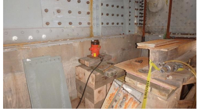
Figure 11: One of the two jacks and cribbing used to restore the bridge to its correct geometry.
