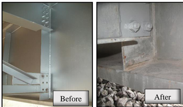
Figure 16: Fatigue Repair (type 3)
