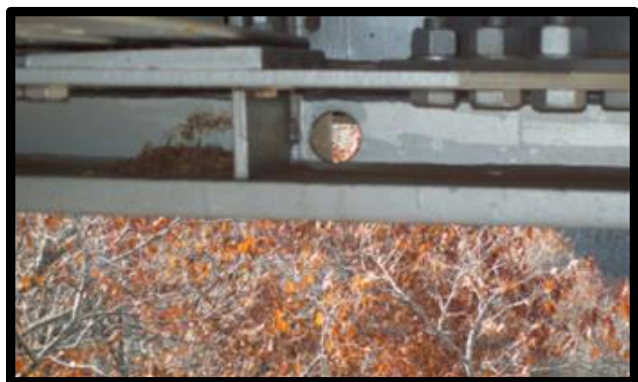
Figure 6: Crack at Web Gap Between Connection Plate of Cross-Frame K-Brace and Gusset Plate Connecting Lateral Lower Bracing
