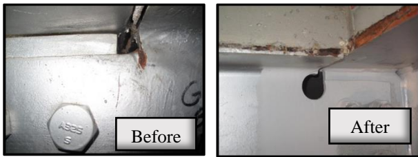
Figure 15: Fatigue Repair (type 2)
