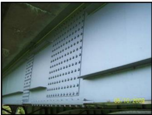
Figure 5: 1991 Web Crack and Bolted Retrofit
