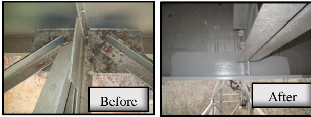
Figure 14: Fatigue Repair (type 1)
