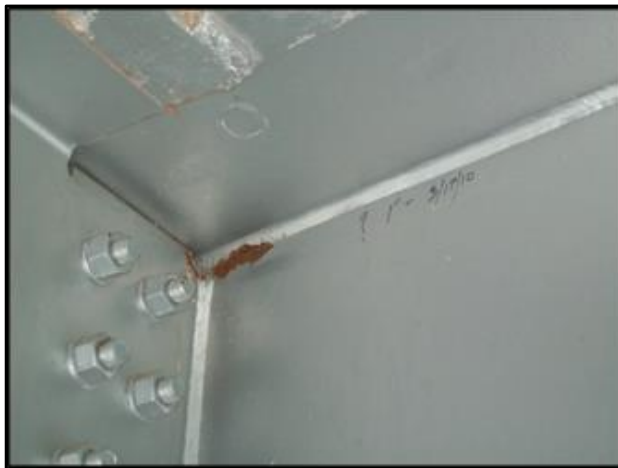
Figure 7: 2009 Cracks at Floorbeams and Delta Girders
