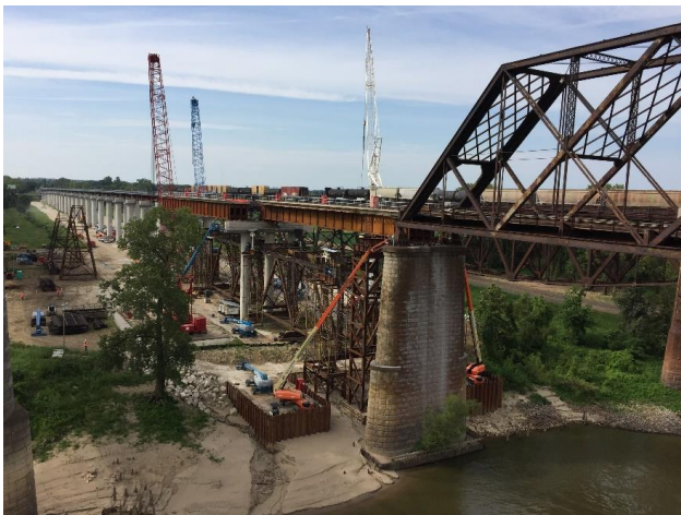
Figure 5: After lowering the 339' deck truss using strand jacks, crews prepare to roll two steel spans during the Phase IV changeout.
